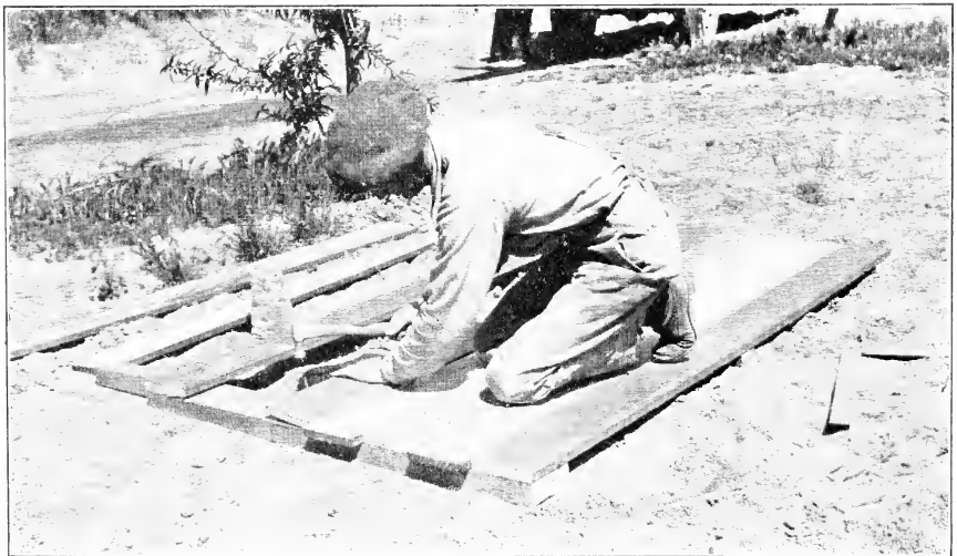
Fig. 7—The side-wall sheathing should be well nailed, and the boards drawn close together.
